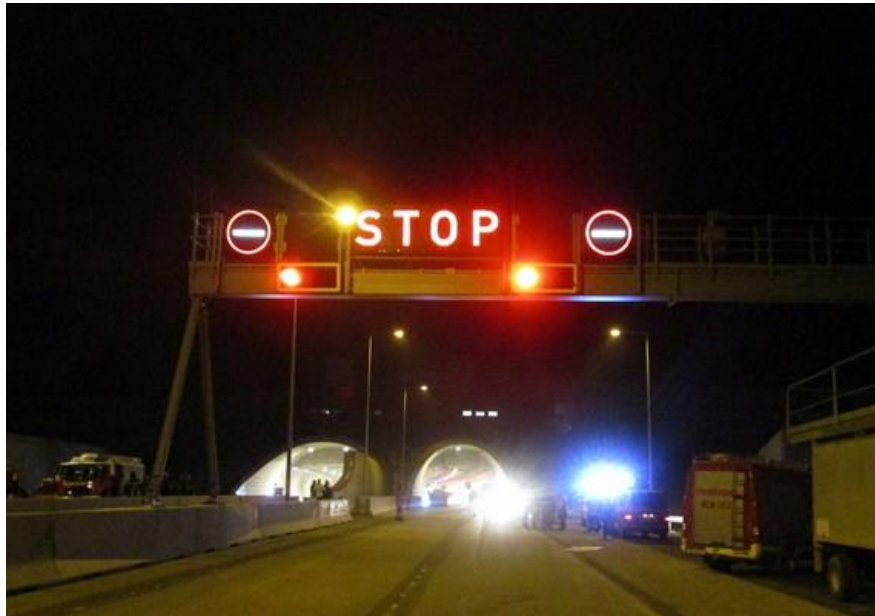
Figure 9: Traffic Signals at Tunnel Portal
