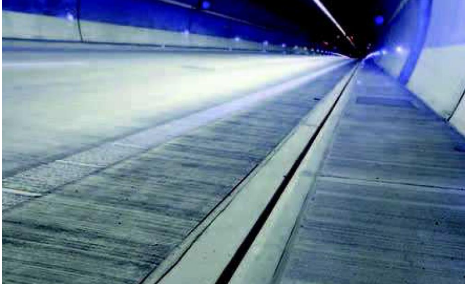
Figure 13 Slotted Channel for Drainage
