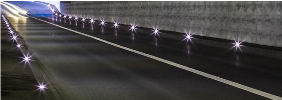
Figure 5: LED Floor Guidance Lights
